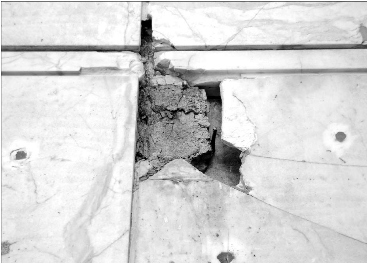
Fig. 1. Marble cladding suffering from failure of original and retrofit connections, as exhibited on a building in Rome (All illustrations by author).
