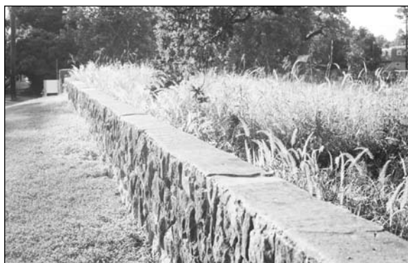
Fig 9. View of the wall along the southern perimeter of the property, June 2010.
