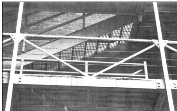
Fig. 8. Exit stair/pedestrian bridge with rusted perimeter, 2006 (Photograph by Baldwin White Architects).
