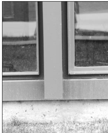
Fig. 15. Enlarged view of original and revised window jamb detail (painted rubber gas-keting), 2008 (Photograph by Robert Whitehead).
